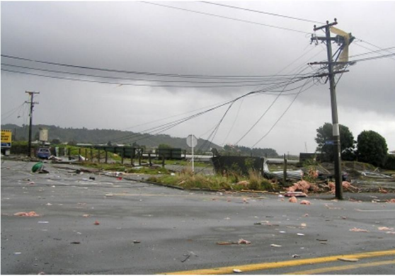
Fig.6. Overhead lines fell down due to strong winds
