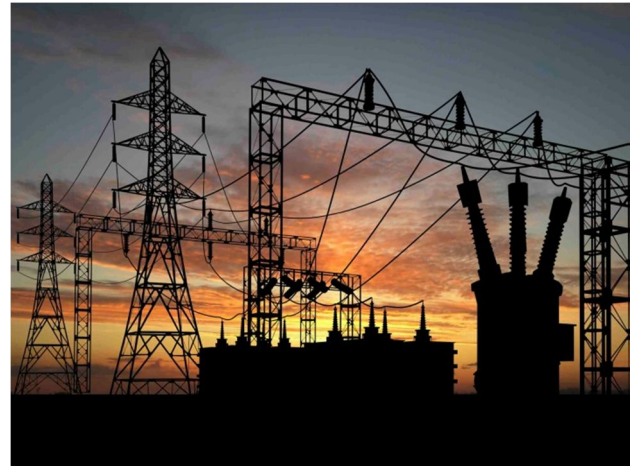
Fig.2. Electrical transmission lines
