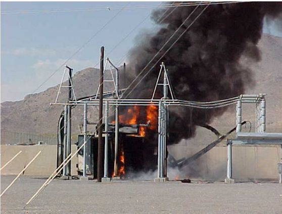
Fig.7. A fire happened in transformer due to electrical fault
