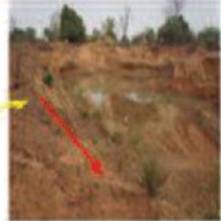
Slope failure around Fuchitako
