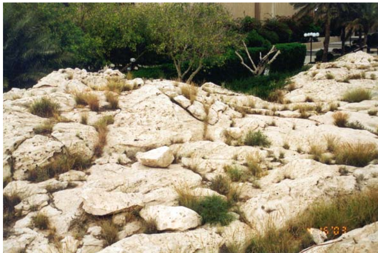
Figure 7: Two photos show the minor local and very localized type fractures within the Dammam dome
