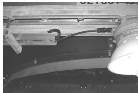
Figure 6 Excess Cable "lost" in Tray
