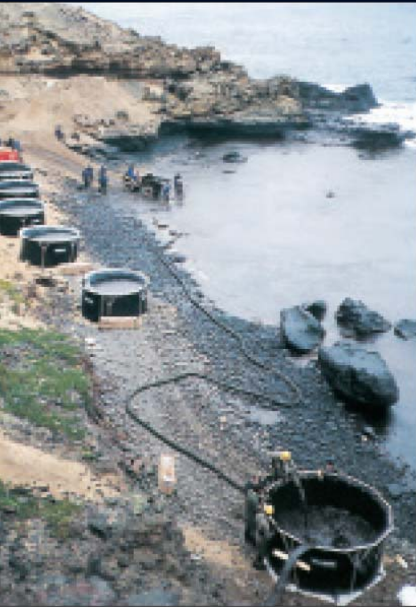
Oil wastes in temporary storage near the shoreline
