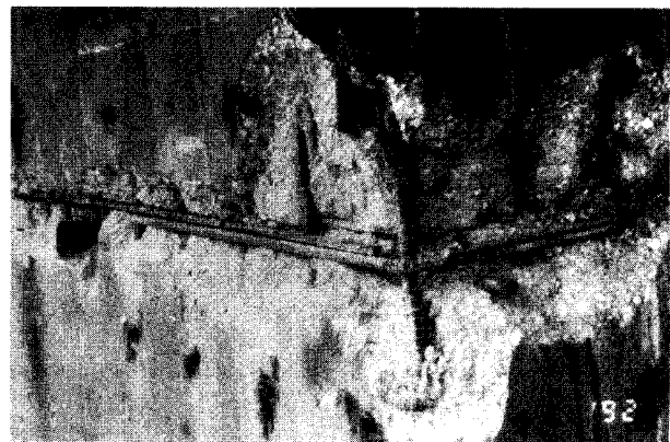
FIG. 1. Damaged Platform/Walls Joints
